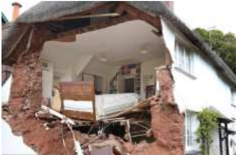
Cement render and other inappropriate finishes can lead to disaster
